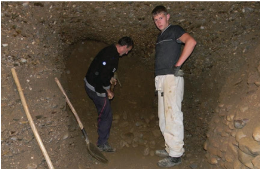
Photo 4; Ravne Tunnels being excavated in 2010. Loose rubble material being removed. A drywall construction retains material blocking side tunnel (right).
