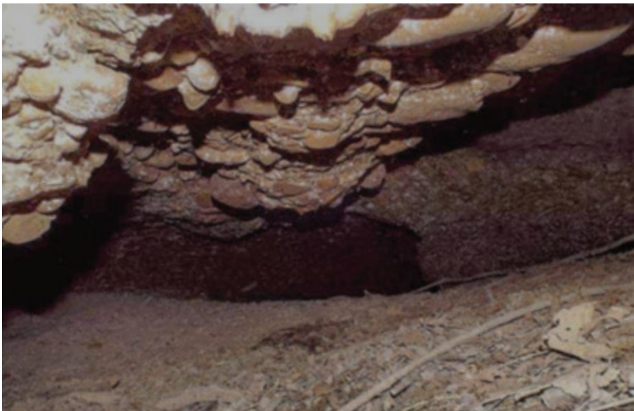
Photo 20; Cavity 'C3'. Looking beyond the excavation face. Removal of disaggregated rubble allowed deeper access into the small cavity at 'C3'. An open chamber, free of filling material is seen beyond the cavities back wall.
