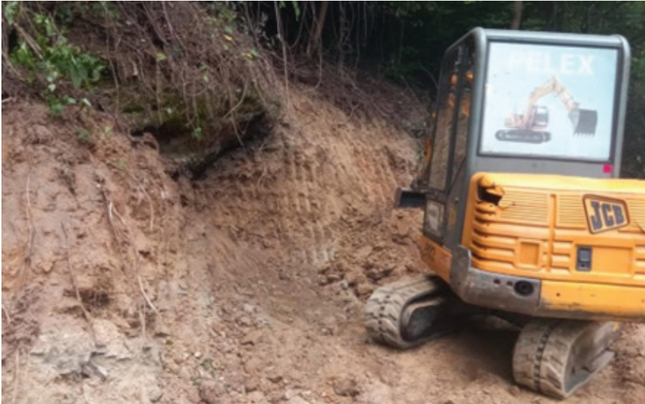
Photo 10; Earthworks being conducted in front of cavity 'C2', removing covering soil and marl layers beneath conglomerate exposure.
