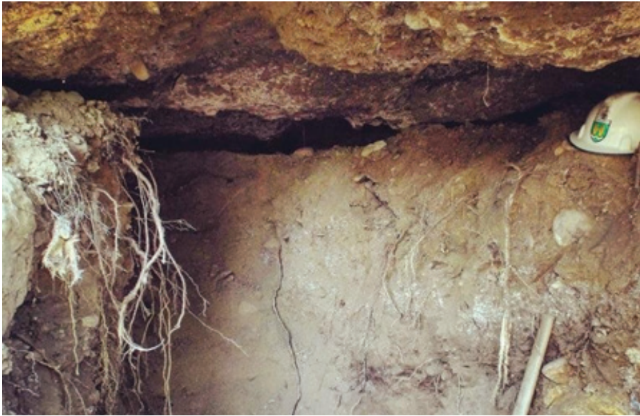
Photo 19; Cavity 'C3' is 15 m north of cavity 'C2'. Image shows cavity 'C3' shortly after removal of rubble from infilled passageway began.
